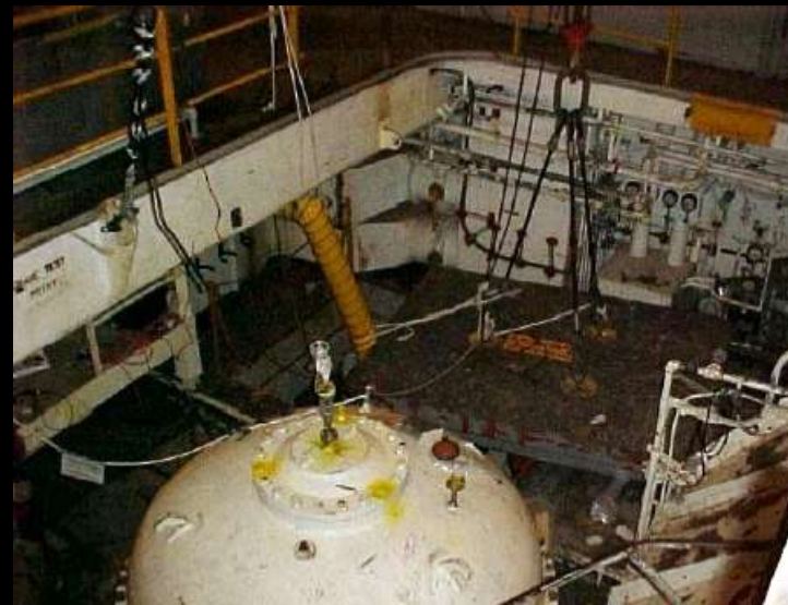
Containment vessel of the MH-1A reactor
